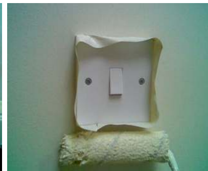
Masking around light switch
