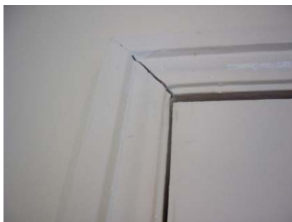
Common type of crack in door frame
