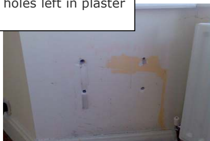
Deep holes left in plaster
