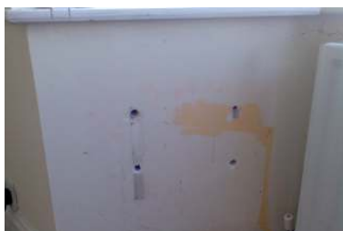
Deep holes left in plaster after radiator was removed
