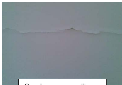
Crack across ceiling
